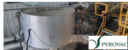
Stirred Tank Reactor
